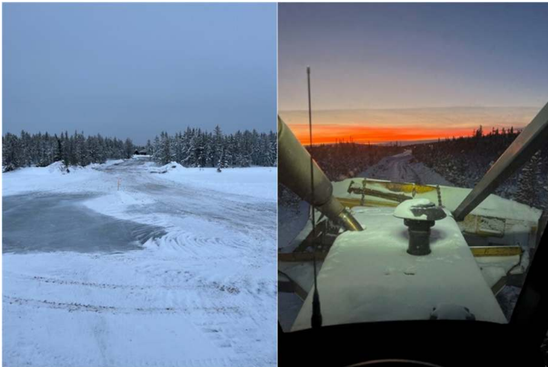
Figure 5 – Access ramp to Lake Ice Road from Base Camp (left) and trail construction (right).
