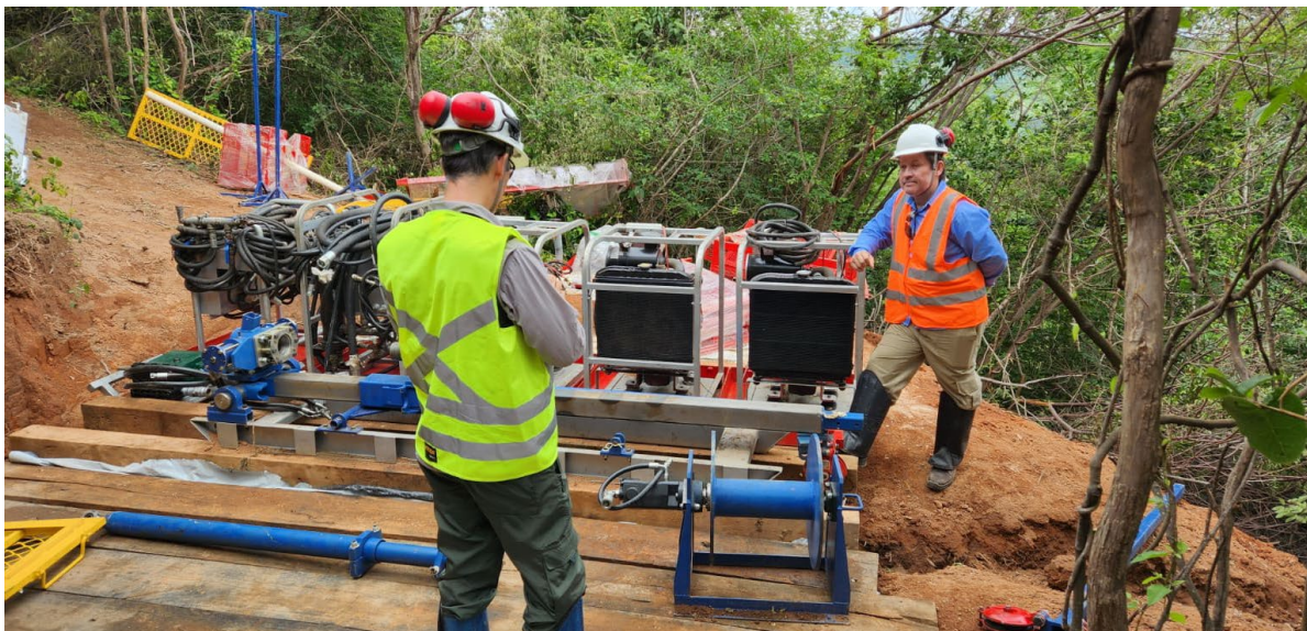
Figure 1: Man portable/ modular diamond drilling rig on site at the Colina Deposit Brazil, capable of drilling to over 400m depth, with minimal environmental impact
