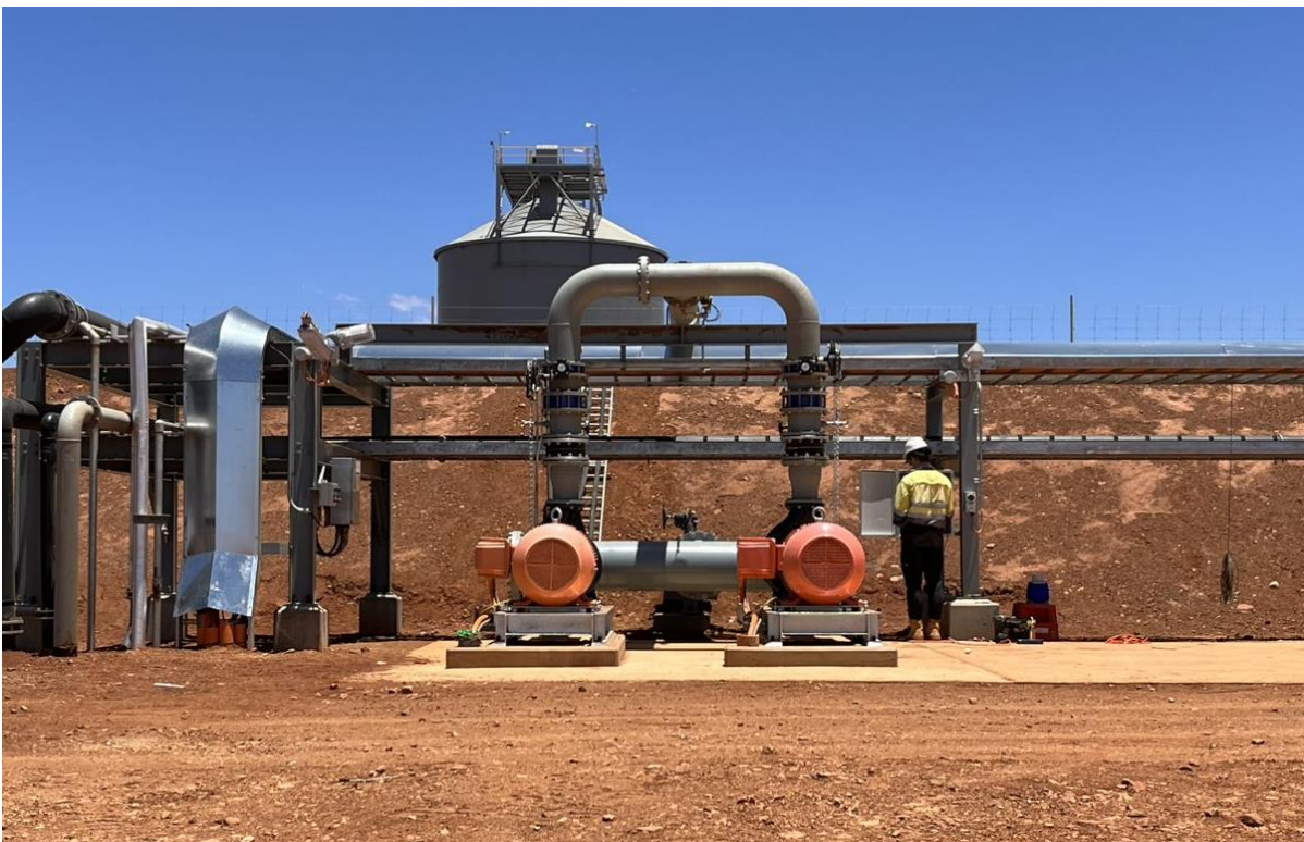
Figure 15 – Water services area pump installation.
