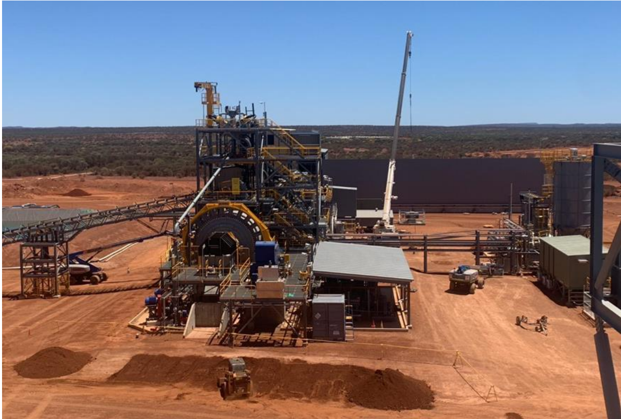
Figure 10 – Ball mill circuit with concentrate shed in the background.
