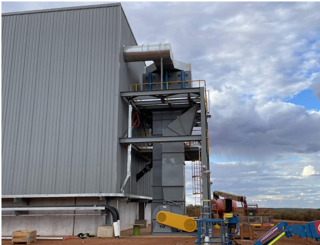
Figure 13 – Concentrate shed Dust Extractor.
