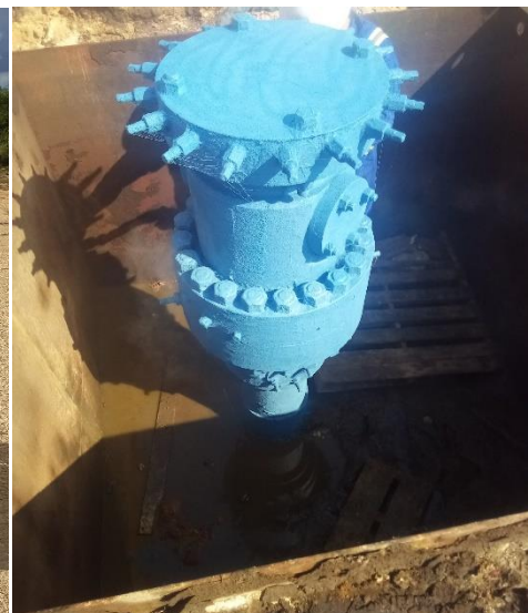
Figure 4 – Zapato-1 well head environmentally sealed
