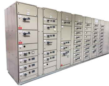
Medium Voltage Distribution
