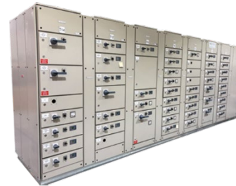
Medium Voltage Distribution
