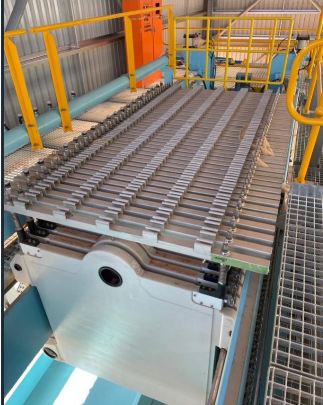
Figure 13 – Concentrate shed filter press.
