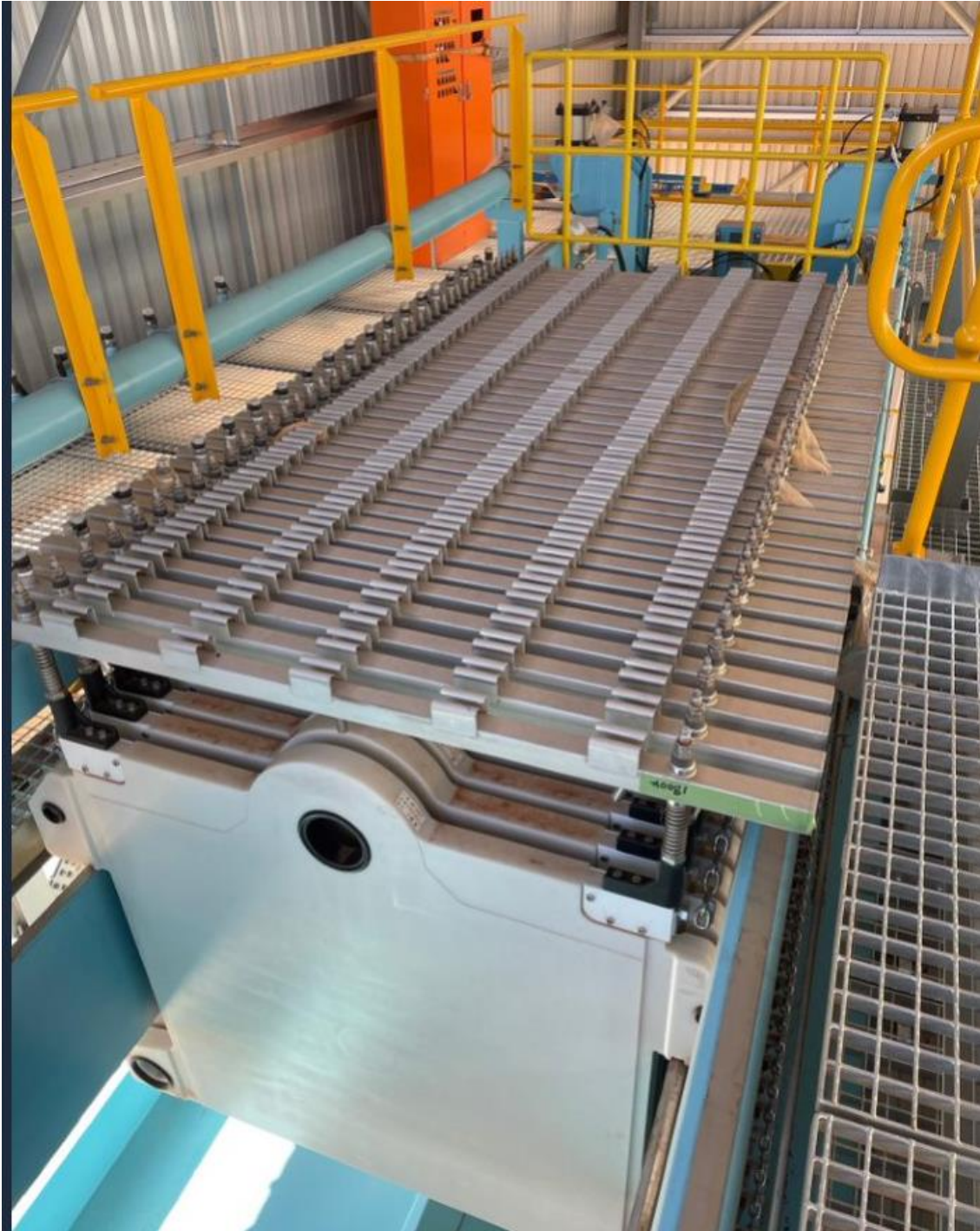
Figure 13 – Concentrate shed filter press.
