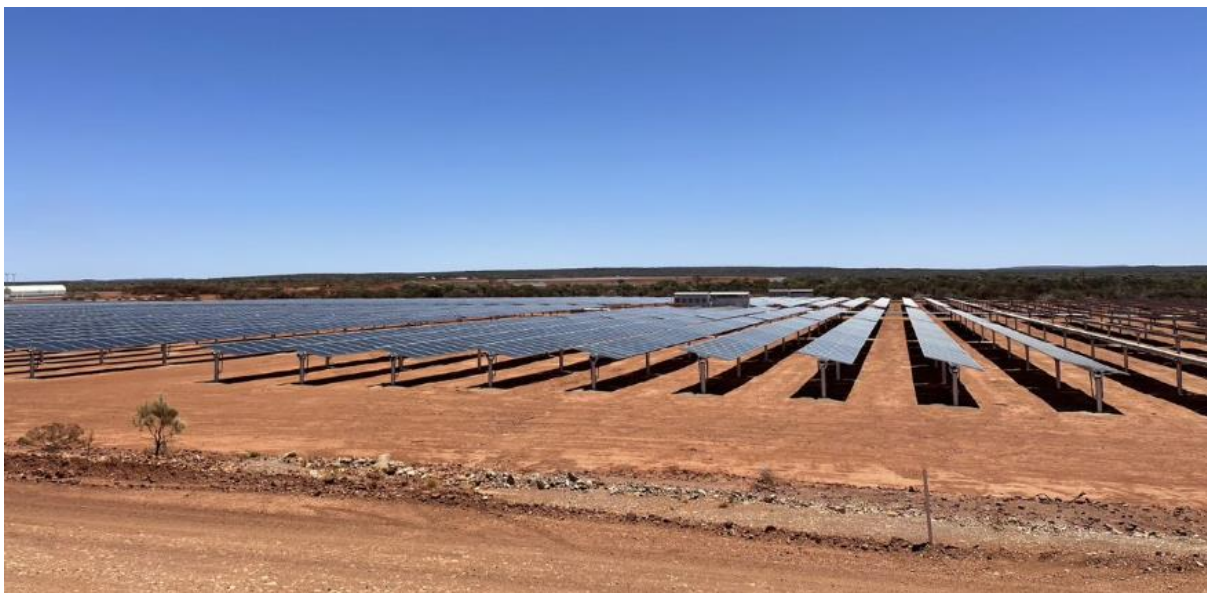
Figure 7 – Abra solar farm has been fully integrated into mines mains power supply (Pacific Energy)
