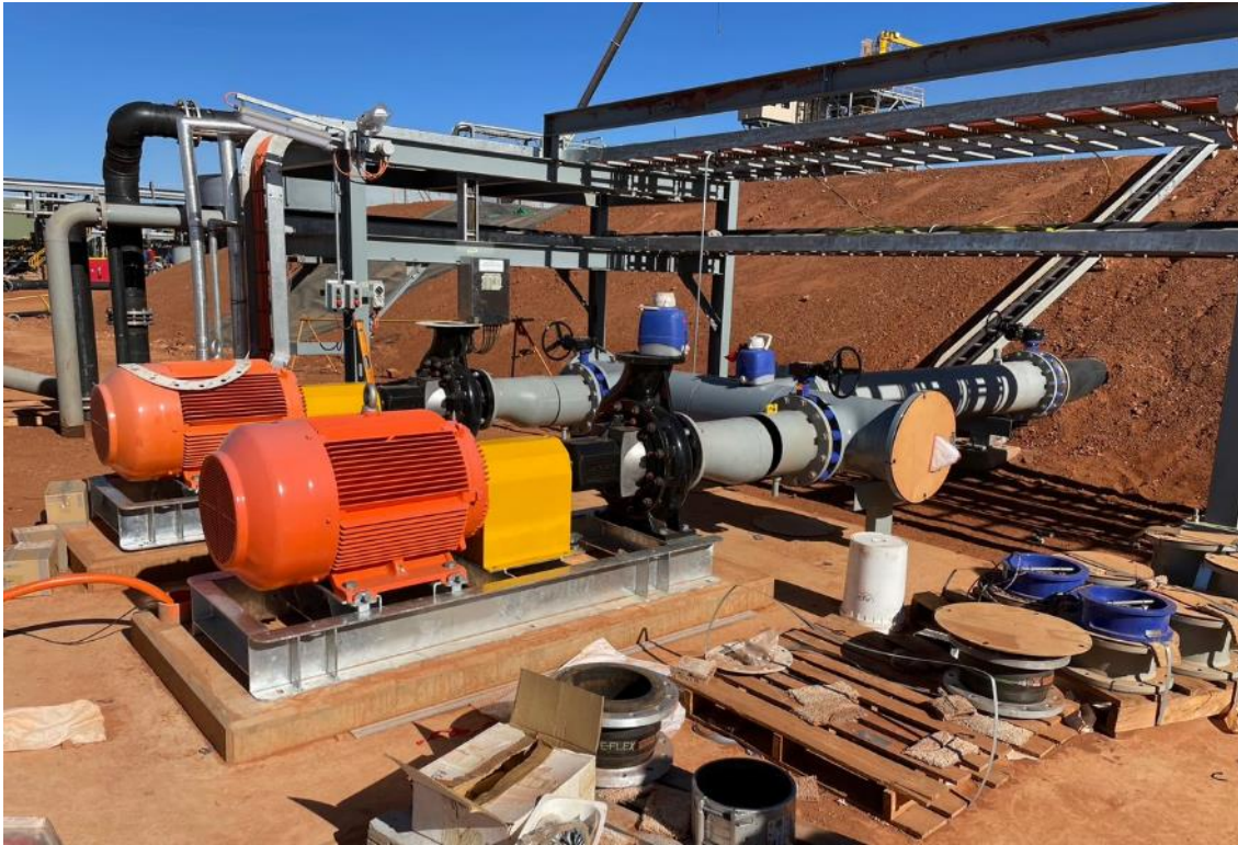
Figure 14 – Water services area pump installation.
