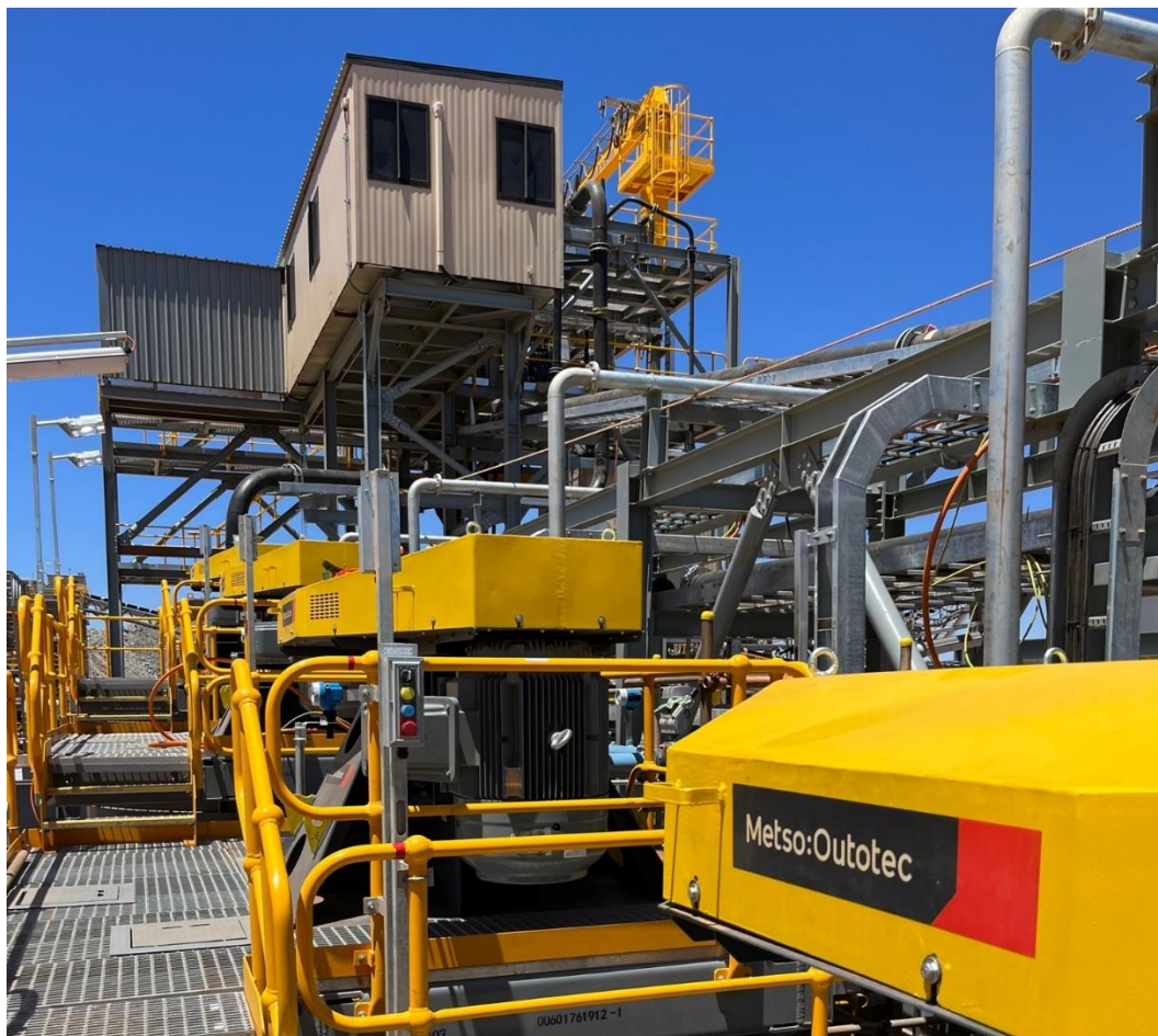
Figure 10 – Mill control above flotation circuit (Photo 11 November).
