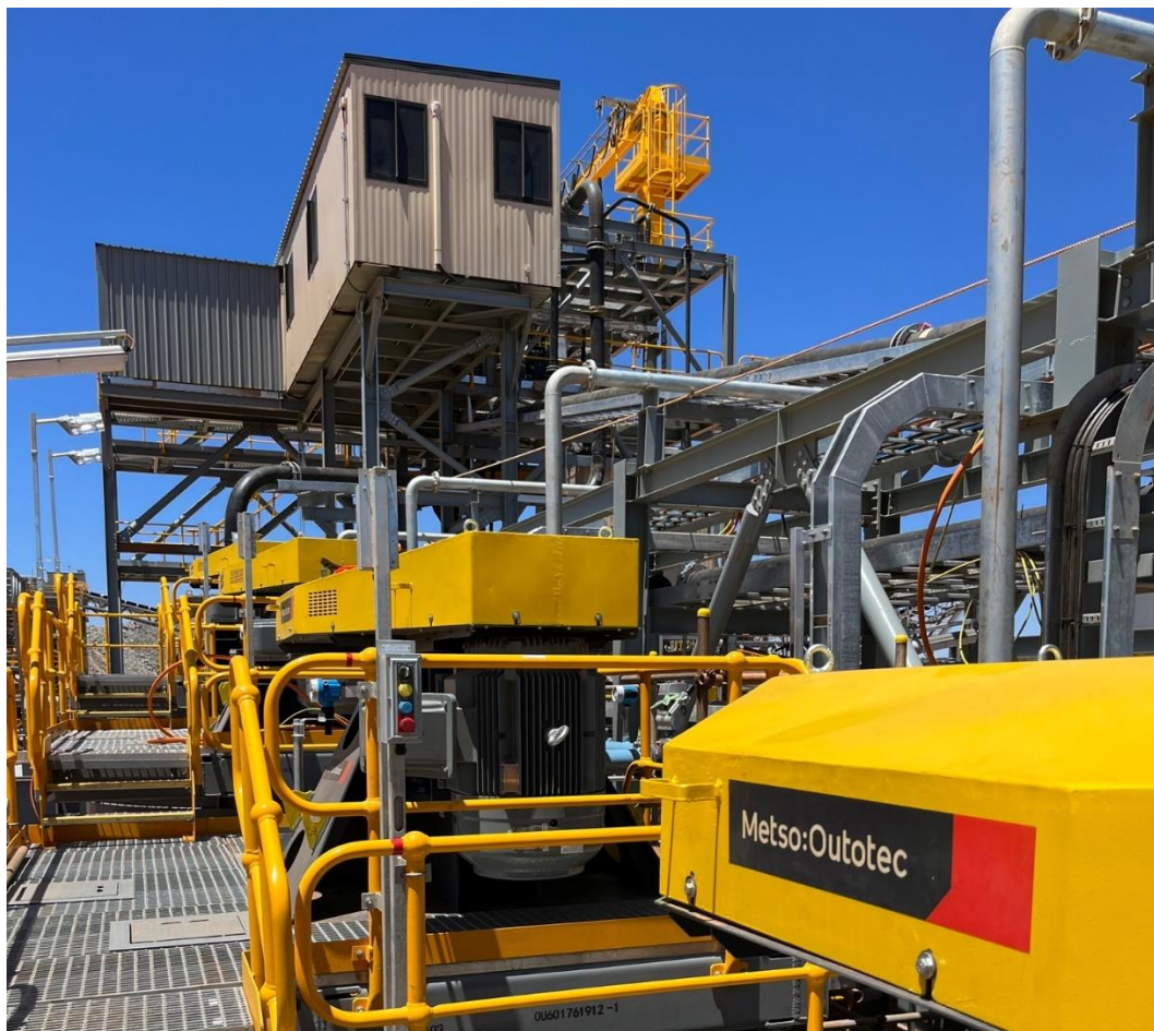
Figure 10 – Mill control above flotation circuit (Photo 11 November).
