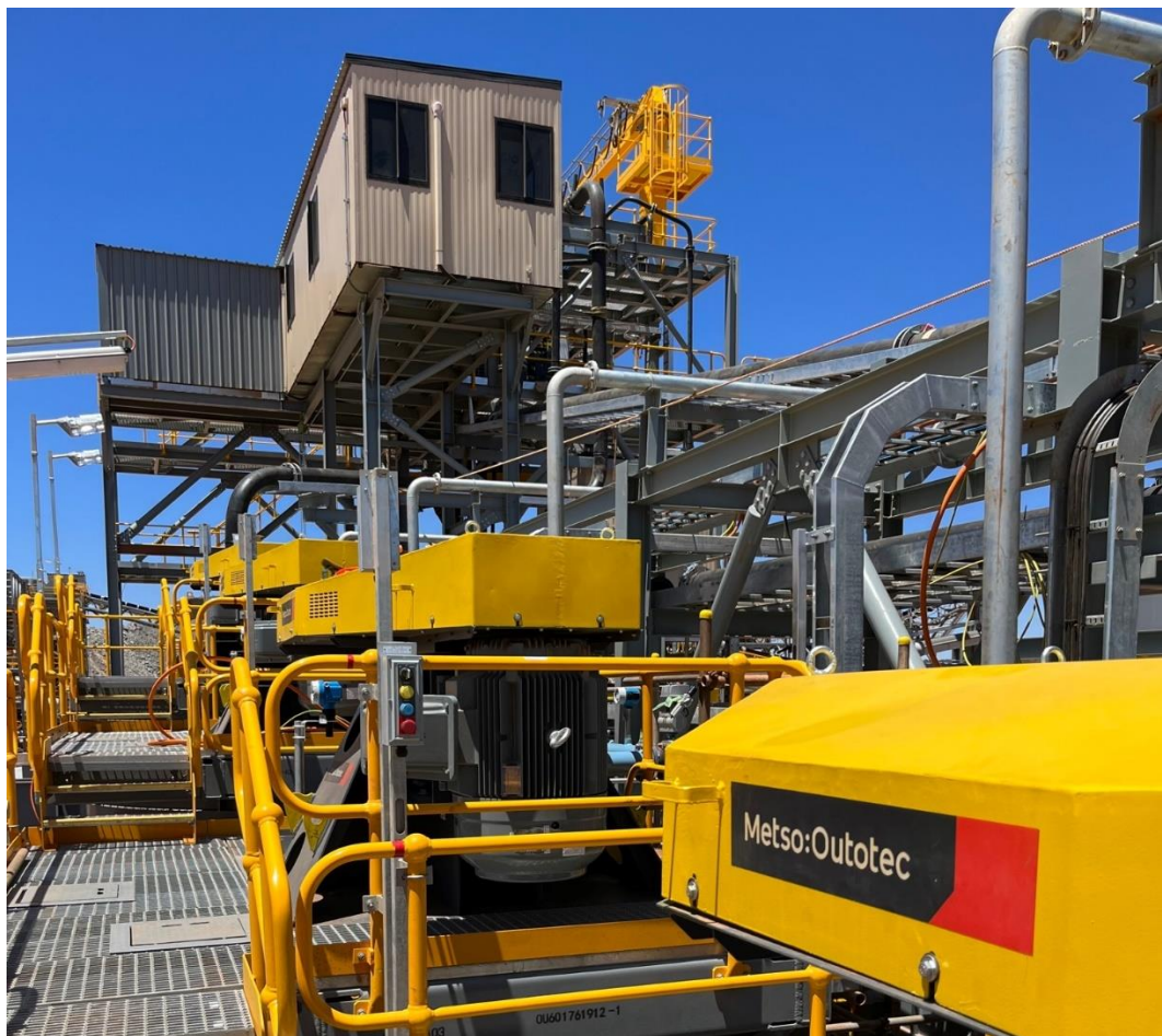
Figure 10 – Mill control above flotation circuit (Photo 11 November).
