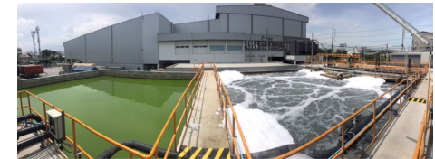
Effluent Treatment Plant in Thailand
