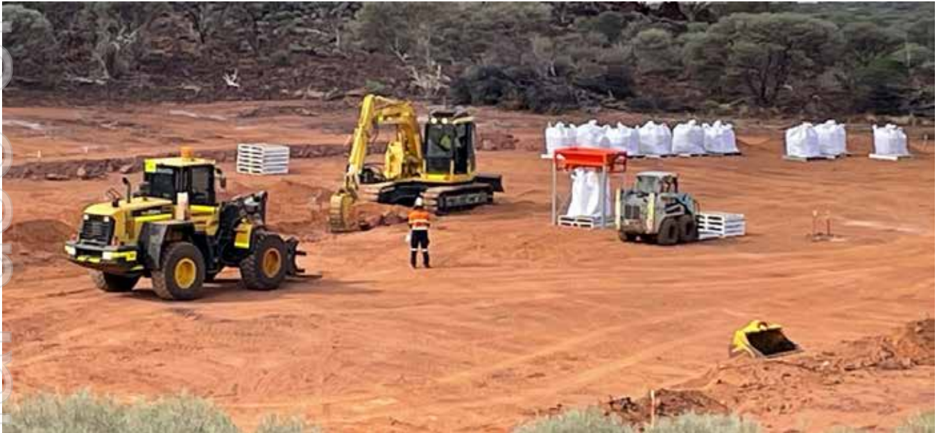
Figure 6 – Costeaming operations to extract, sample and bag mineralisation at Barrambie. Source: Neometals.
