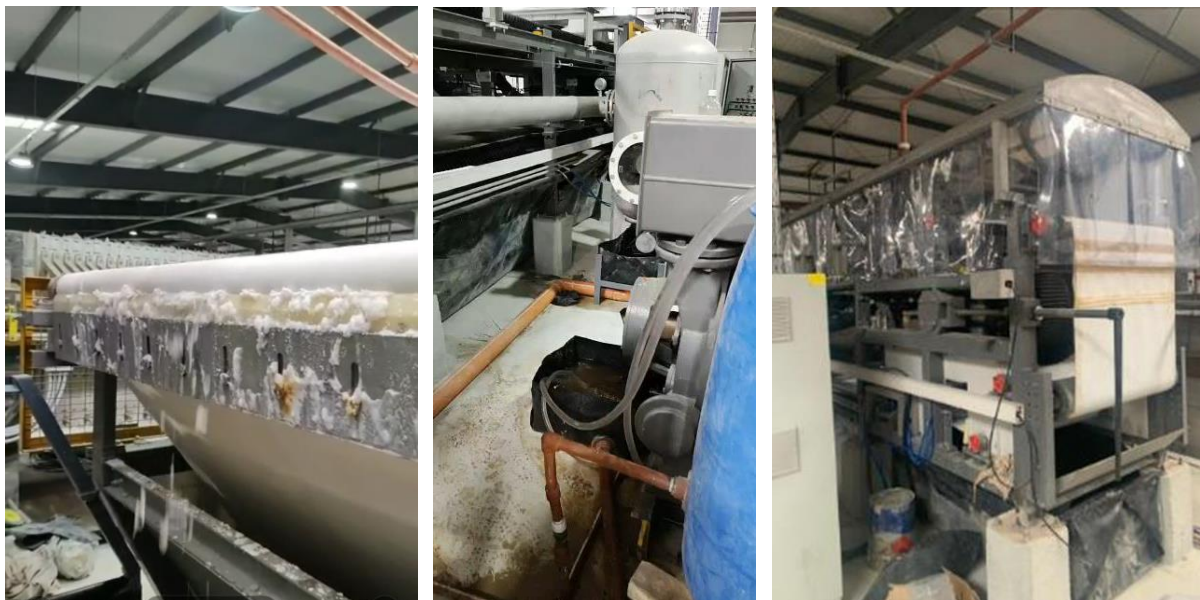
Figures 1-3. Rincon Lithium Project – 2,000tpa Operation Commissioning & Production Test-Works
