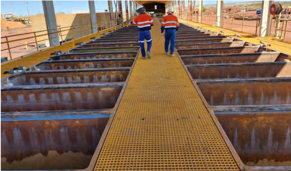
Image 8 / EW cells stripped of anodes and cathodes, cleaned and hydrotested waiting for refurbishment
