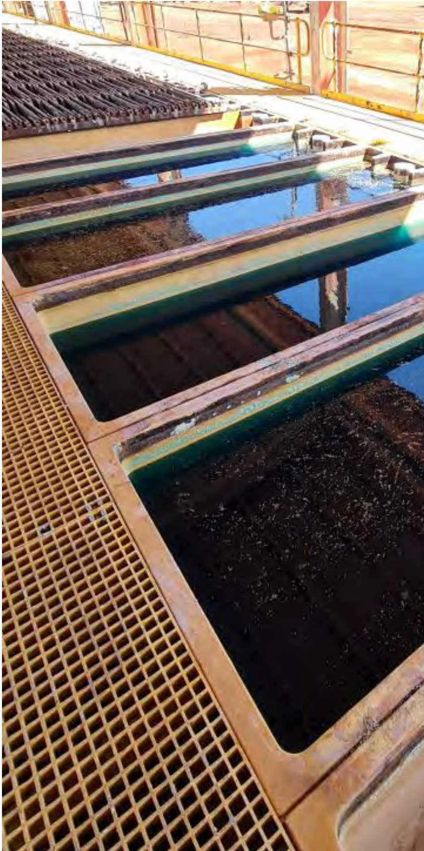
Image 7 / Hydro testing EW cells following removal of cathodes and anodes and clean up
