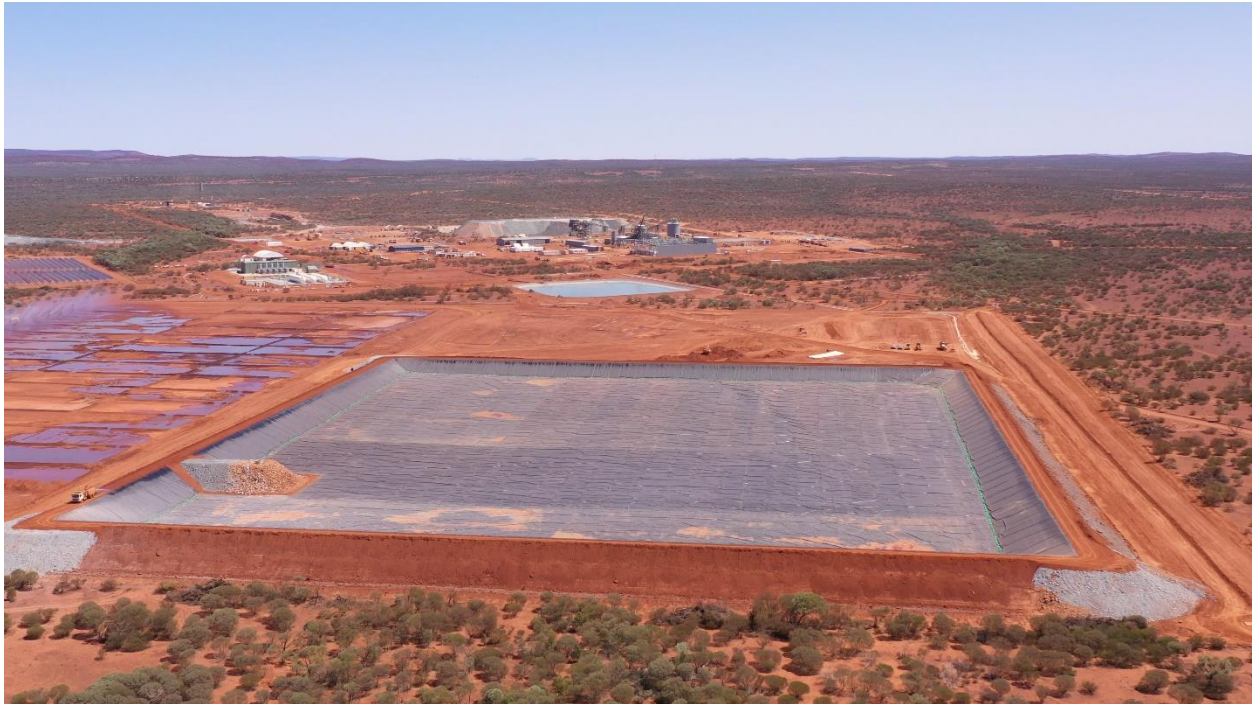
Figure 7. Completed TSF (stage 1) with Abra plant in background and showing mine dewatering evaporation (Photo – 14 October 2022).
