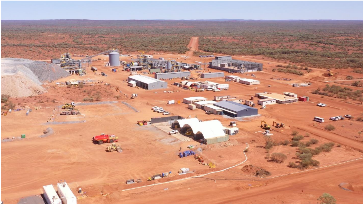
Figure 5. Work progress at the main Abra plant and infrastructure area looking West (Photo – 14 October 2022).
