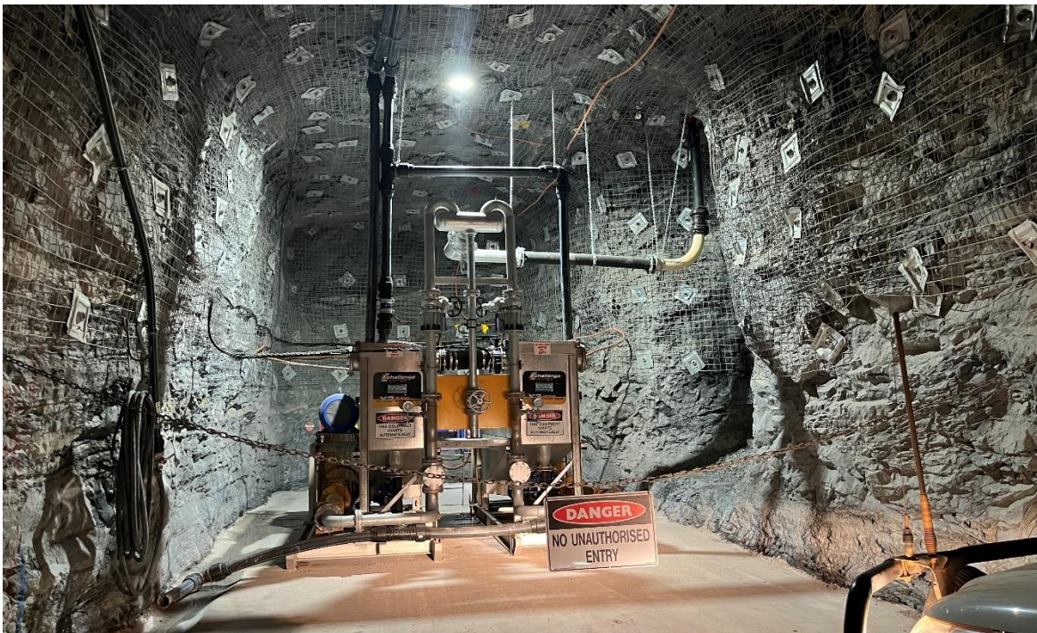
Figure 12. Underground pump station (Photo 30 September 2022).
