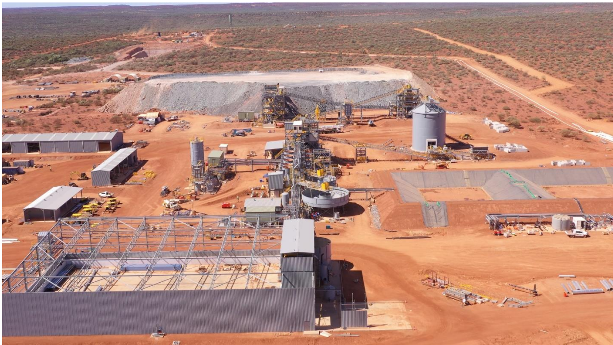
Figure 6. Work progress at the main Abra plant and infrastructure area looking South with mine box-cut and paste plant construction site in the background (Photo – 14 October 2022).
