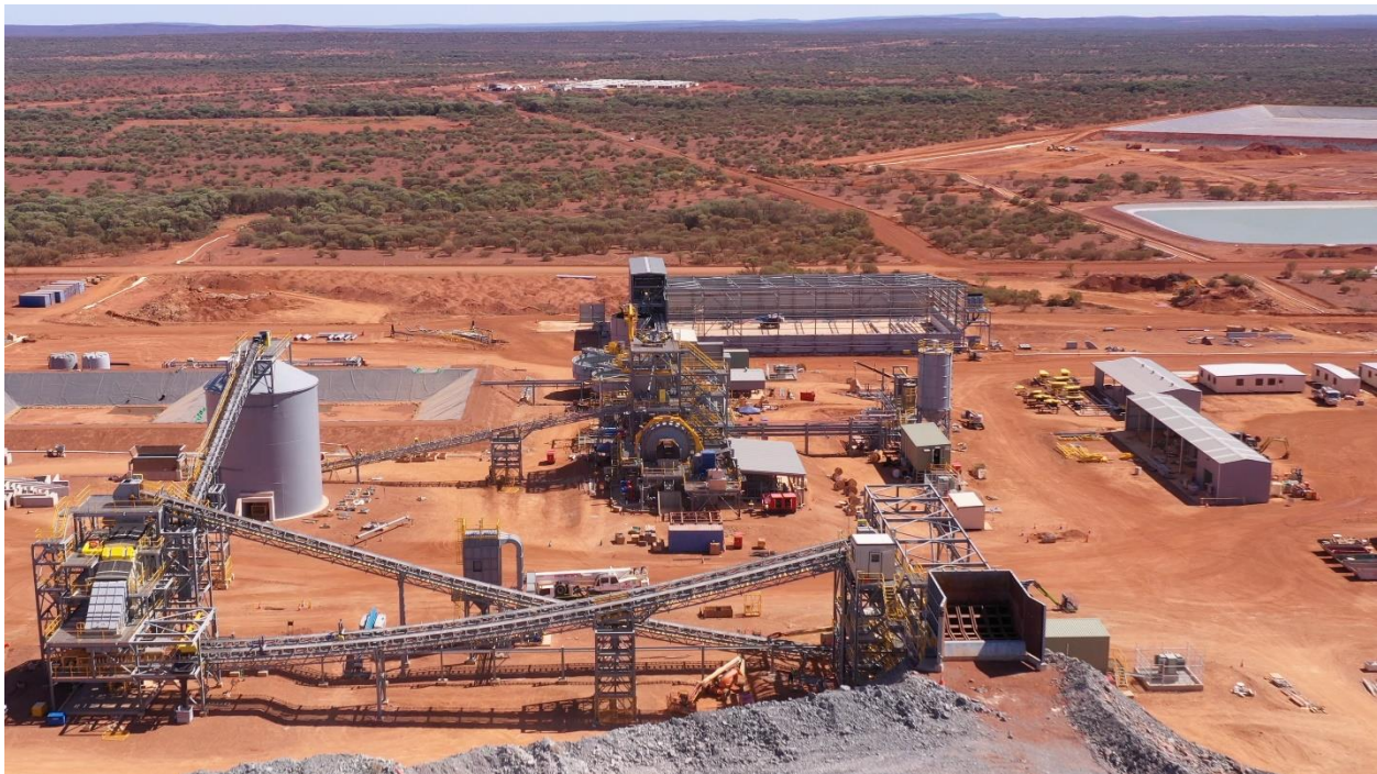
Figure 4. Abra processing plant progress in early October with TSF and village seen in the background (Photo – 14 October 2022).
