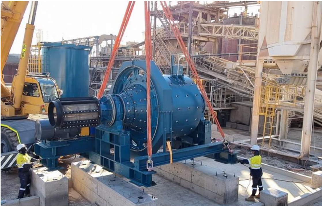
Figure 4: Refurbished Lime Slaking Mill for Wiltails
