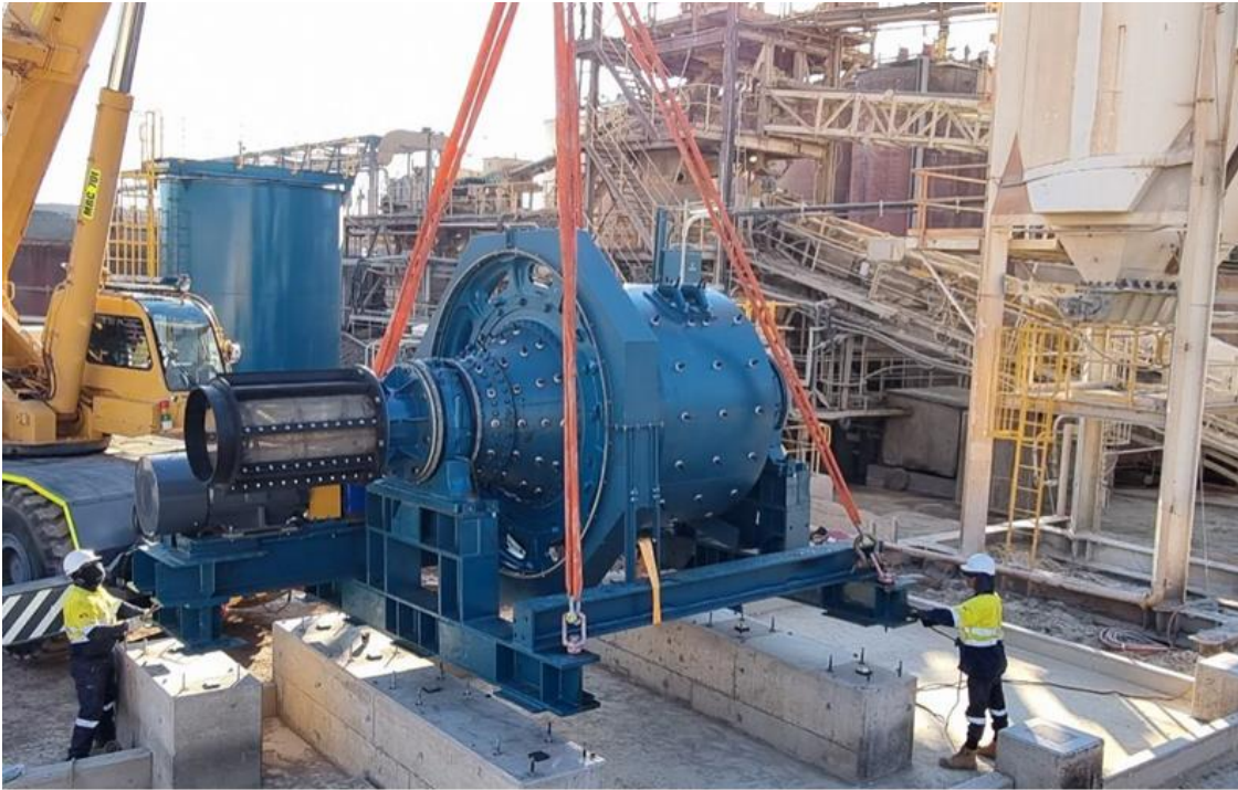
Figure 4: Refurbished Lime Slaking Mill for Wiltails
