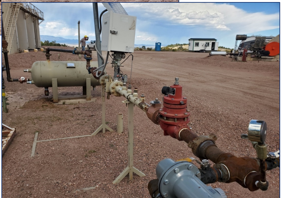
Figure 3 Gas feed from Pathfinder well to gas-fired generators.
