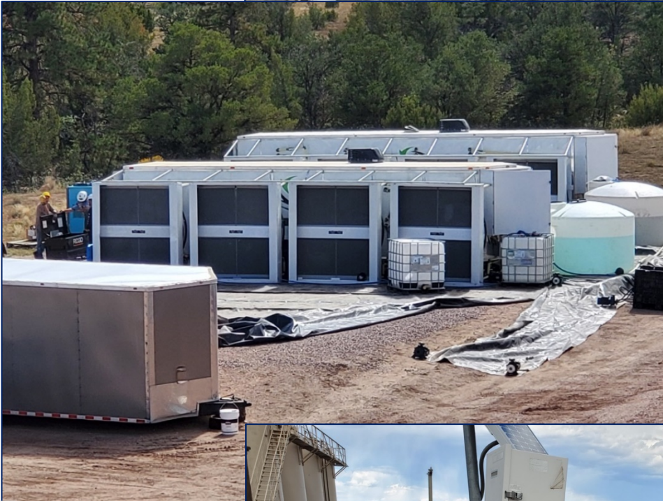
Figure 2 First 2 EMUs fully installed, commissioned and operating.
