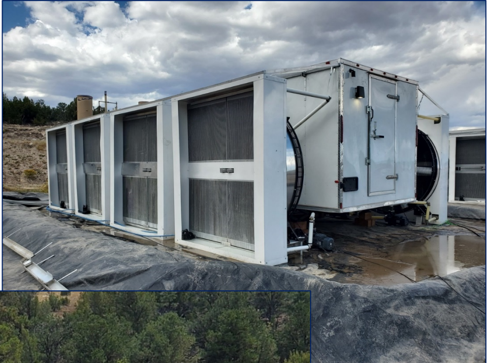
Figure 1 Cooling Modules Installed at Elite Mobile Unit
