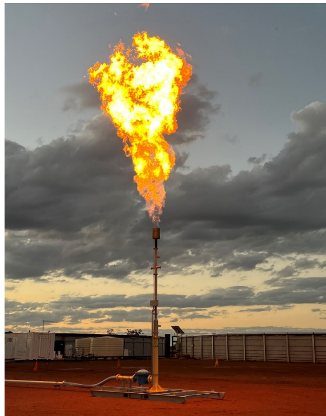
Figure 1 – Mahalo North 1 flare
