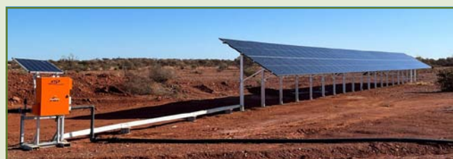
Borefield powered by a solar array.
