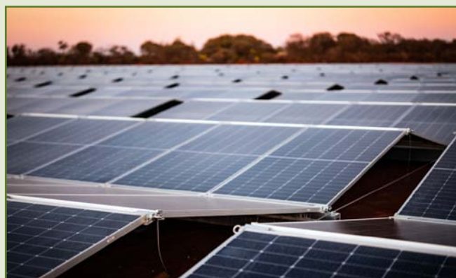
Solar farm at KOTH providing 2MW to the operation.
