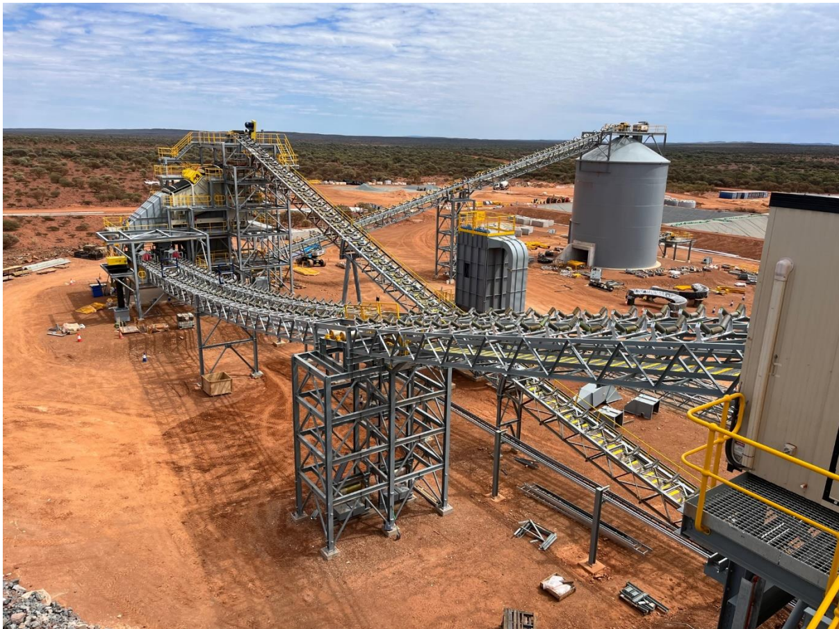
Figure 1 – Abra plant screening and materials handling (photo: 9 September).
