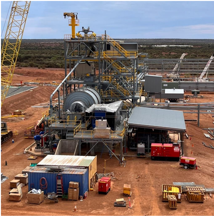
Figure 8 – Abra mill Flotation and concentrate areas (photo 9 September).
