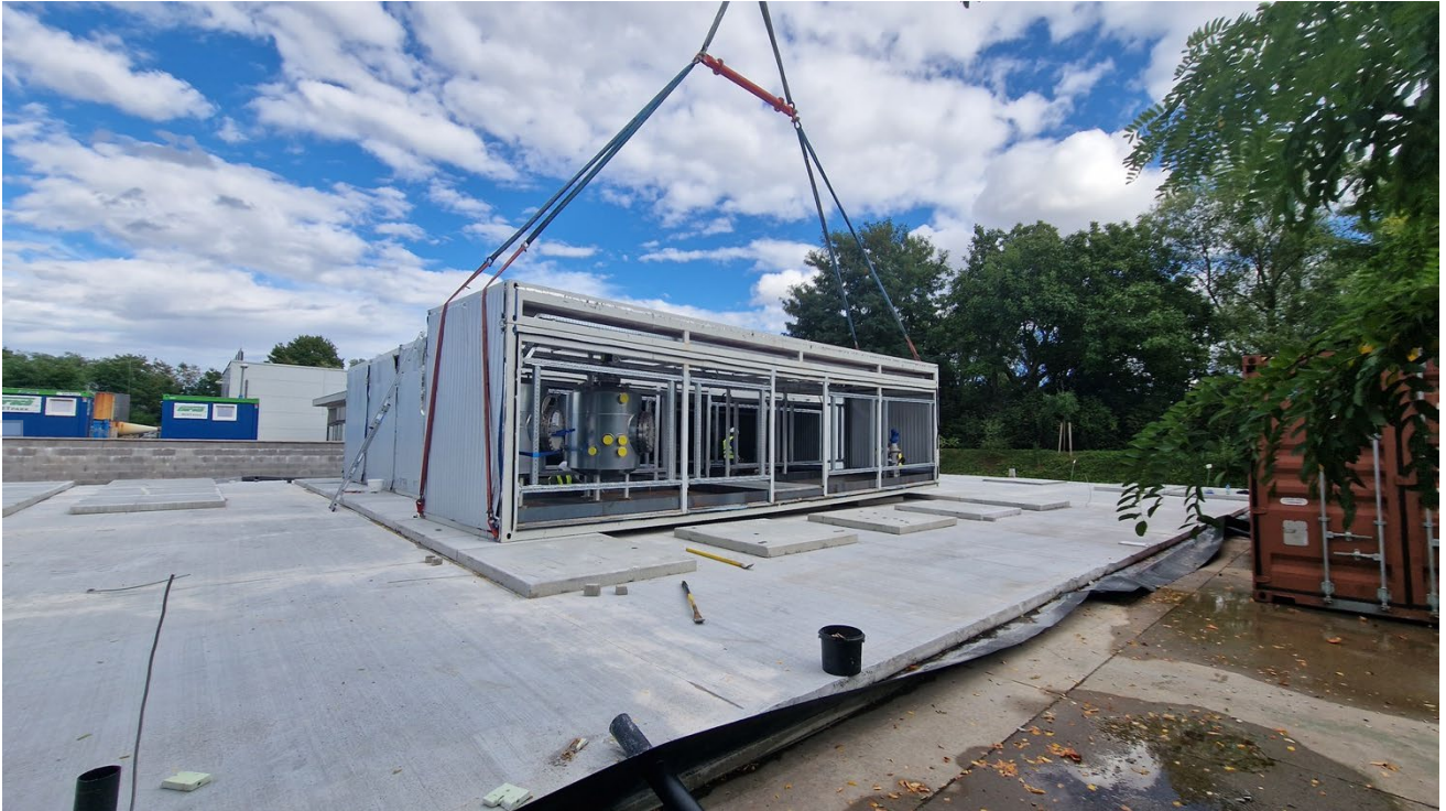
Positioning of the prefabricated containers at the Sorption-Demo Plant in Landau, Germany.
