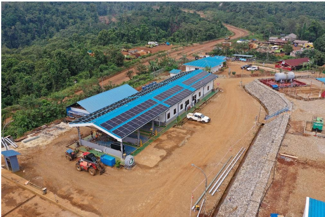
The existing 396kWp plus 250kWh battery storage project at the Hengjaya Mine
