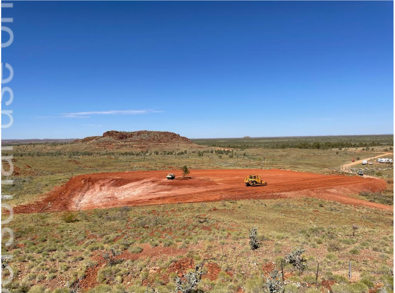
Figure 10. Exploration camp construction underway with levelling and compaction of 70m x 70m area in preparation for dome-sheltered core yard, accommodation, ablution block, workshop and offices. The prominent hill in the background is the part of the Main Hill prospect. View looking south.
