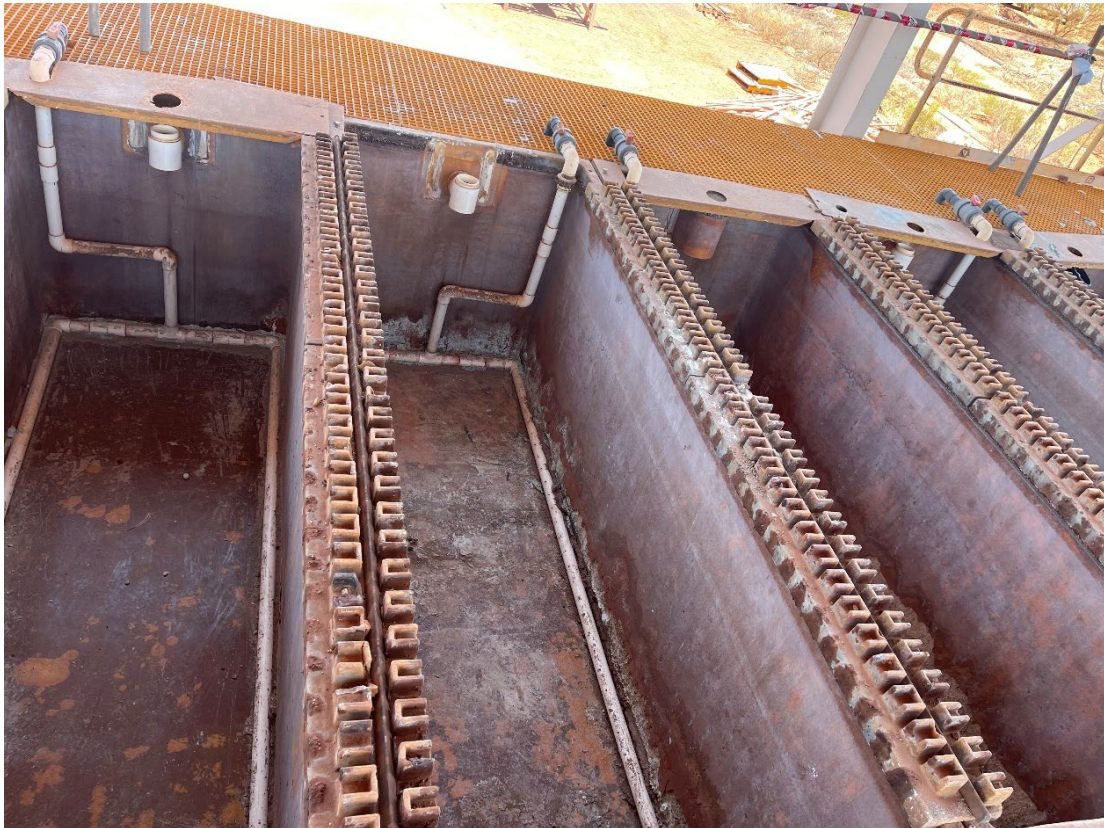
Image 9 / Cleaned EW Cells ready for condition inspection
