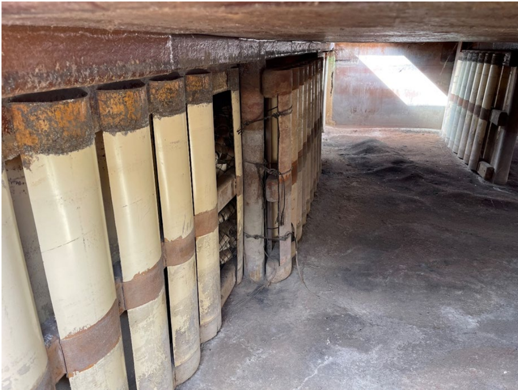
Image 3 / SX Mixer Settler cleanout lower level
