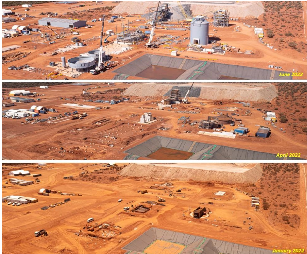
Figure 3. Work progress from January 2022, through April 2022 to June 2022 at the main Abra plant and infrastructure area looking South.
