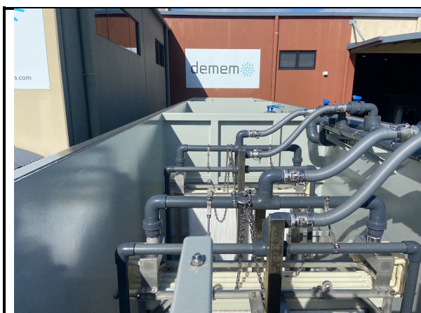
De.mem containerized waste water treatment system (1)
