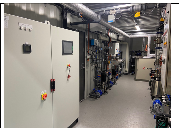
De.mem containerized waste water treatment system (2)
