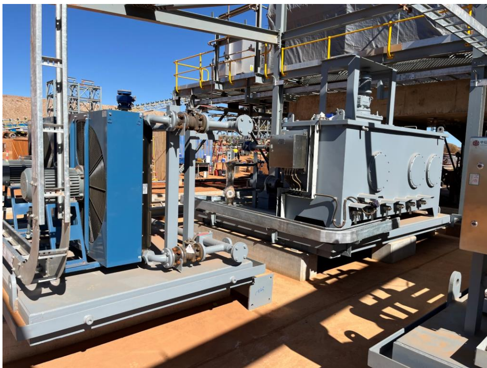
Figure 6 – Mill bearing lubrication equipment (photo: 12 July).
