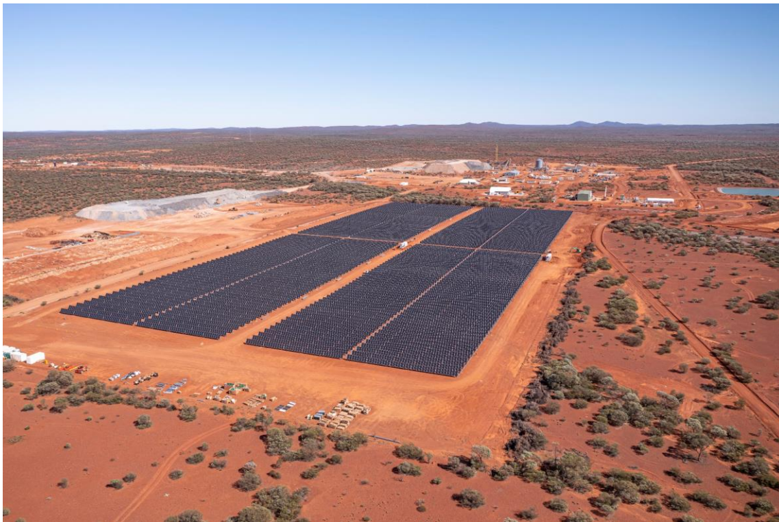
Figure 14 – Abra site installed solar panels.
