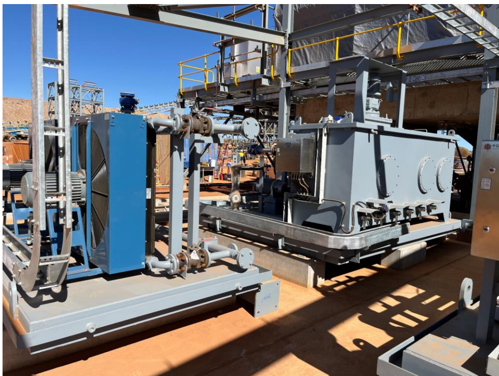
Figure 6 – Mill bearing lubrication equipment (photo: 12 July).
