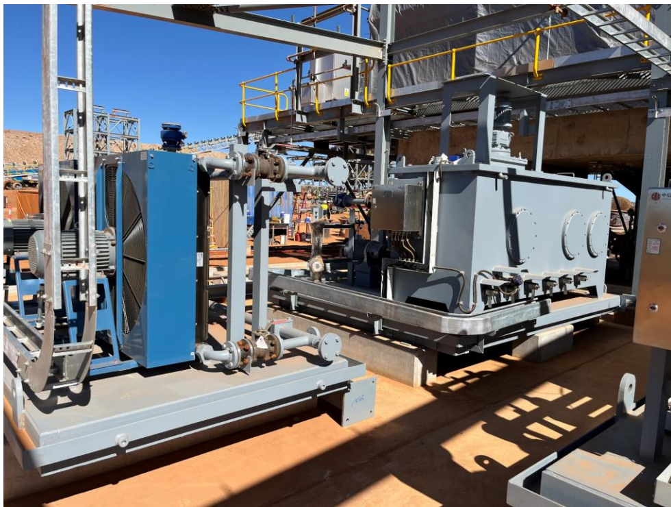
Figure 6 – Mill bearing lubrication equipment (photo: 12 July).
