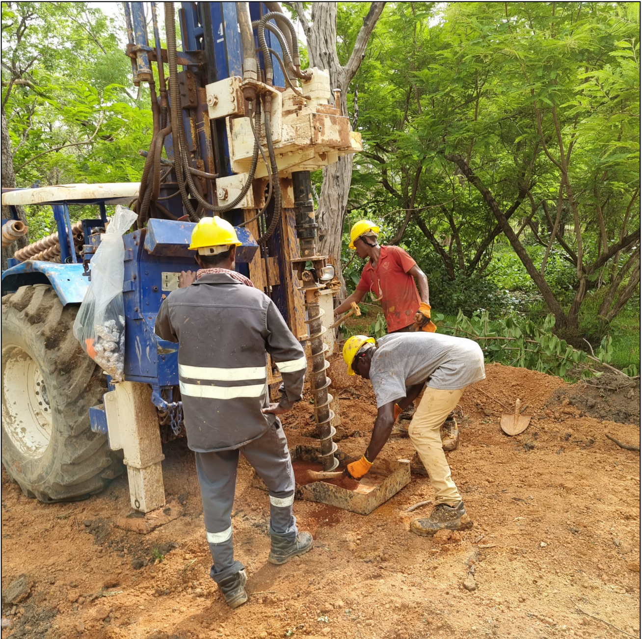
Figure 4: Infill auger drilling on the Kada Gold Project at Bereko Prospect, 7km north of the ~930,000oz Mineral Resource area at Massan Prospect.
