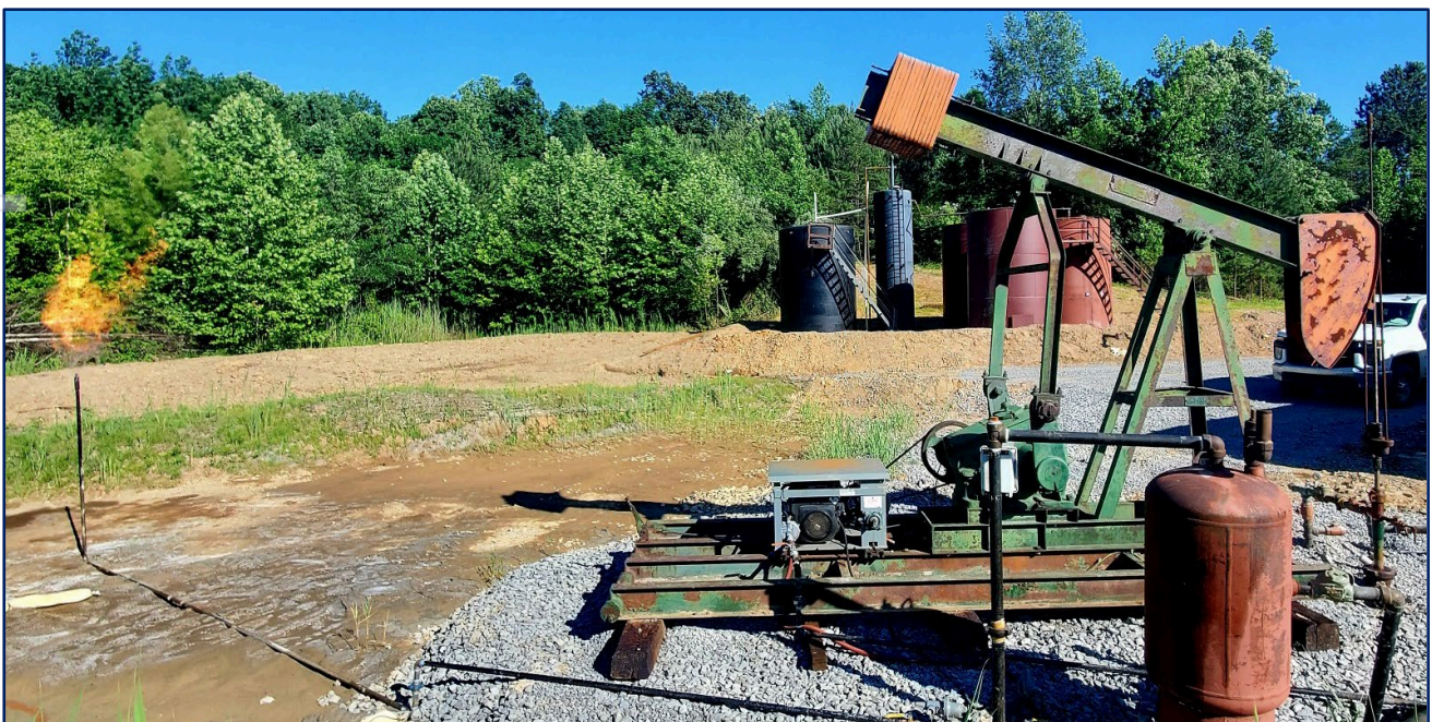
DPI-2605 PUMP, TANK BATTERY & GAS FLARE: LOW-COST PRODUCTION INFRASTRUCTURE
