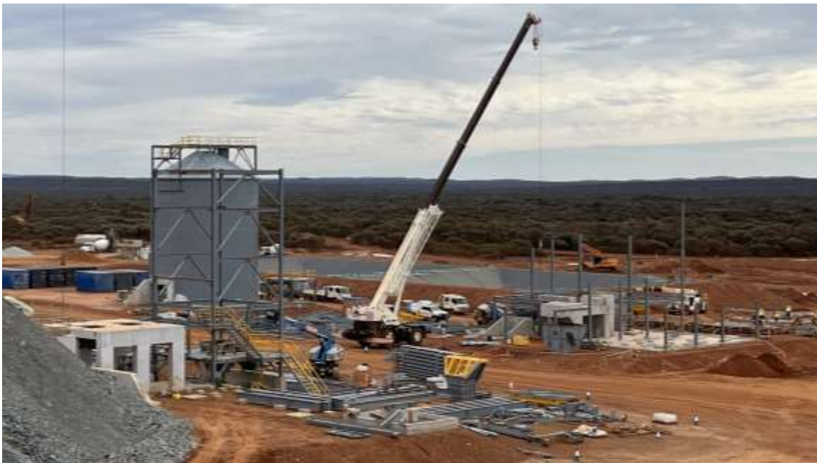
Figure 1 shows the Abra processing plant construction activities in May 2022. Commencement of structural steel installation for the crusher and mill areas in front of the completed fine ore bin (FOB).
