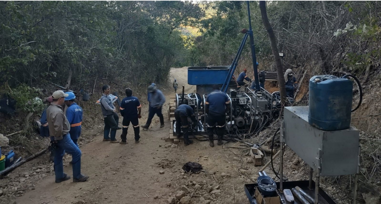
Figure 6: Establishment and drill-rig set-up of drillhole MADD003, Monte Alto Prospect – Salinas Lithium Project, Brazil
