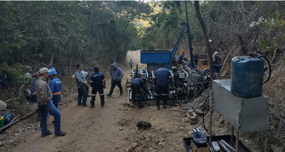
Figure 6: Establishment and drill-rig set-up of drillhole MADD003, Monte Alto Prospect – Salinas Lithium Project, Brazil
