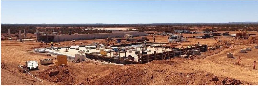
Figure 8 – Concentrate thickener area with concentrate shed in the background.
