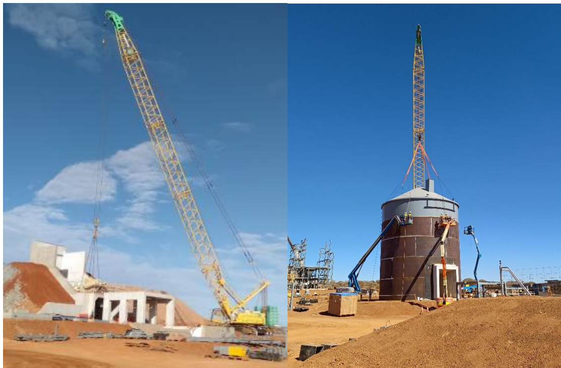
Figure 1 – Lifting of the primary jaw crusher and fine ore bin top into position.
