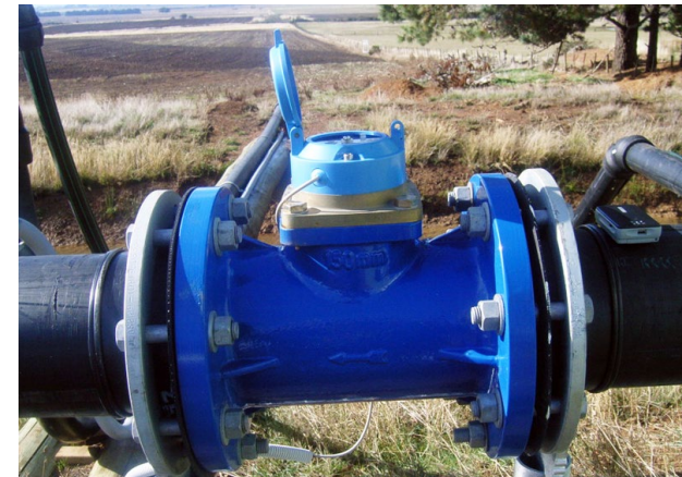
^ Photo: Water Meter Used to prevent theft of water Often utilises tamper proof technology
