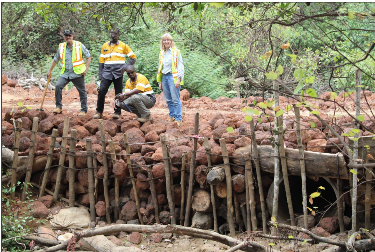
Figure 14: Traditional laterite bridge which provides access from Gogbala to Tchaga during the wet season
