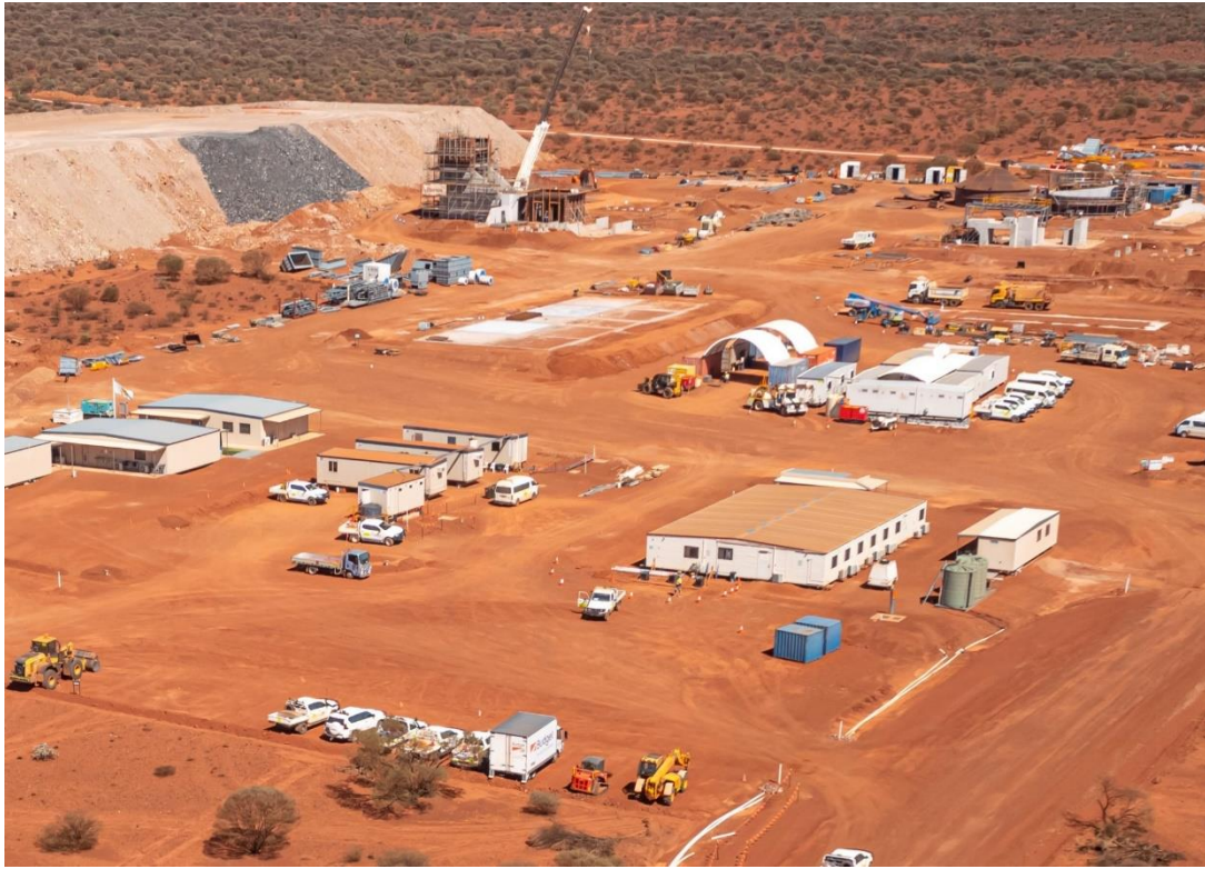
Figure 4. Work progress at the main Abra plant and infrastructure area looking West.
