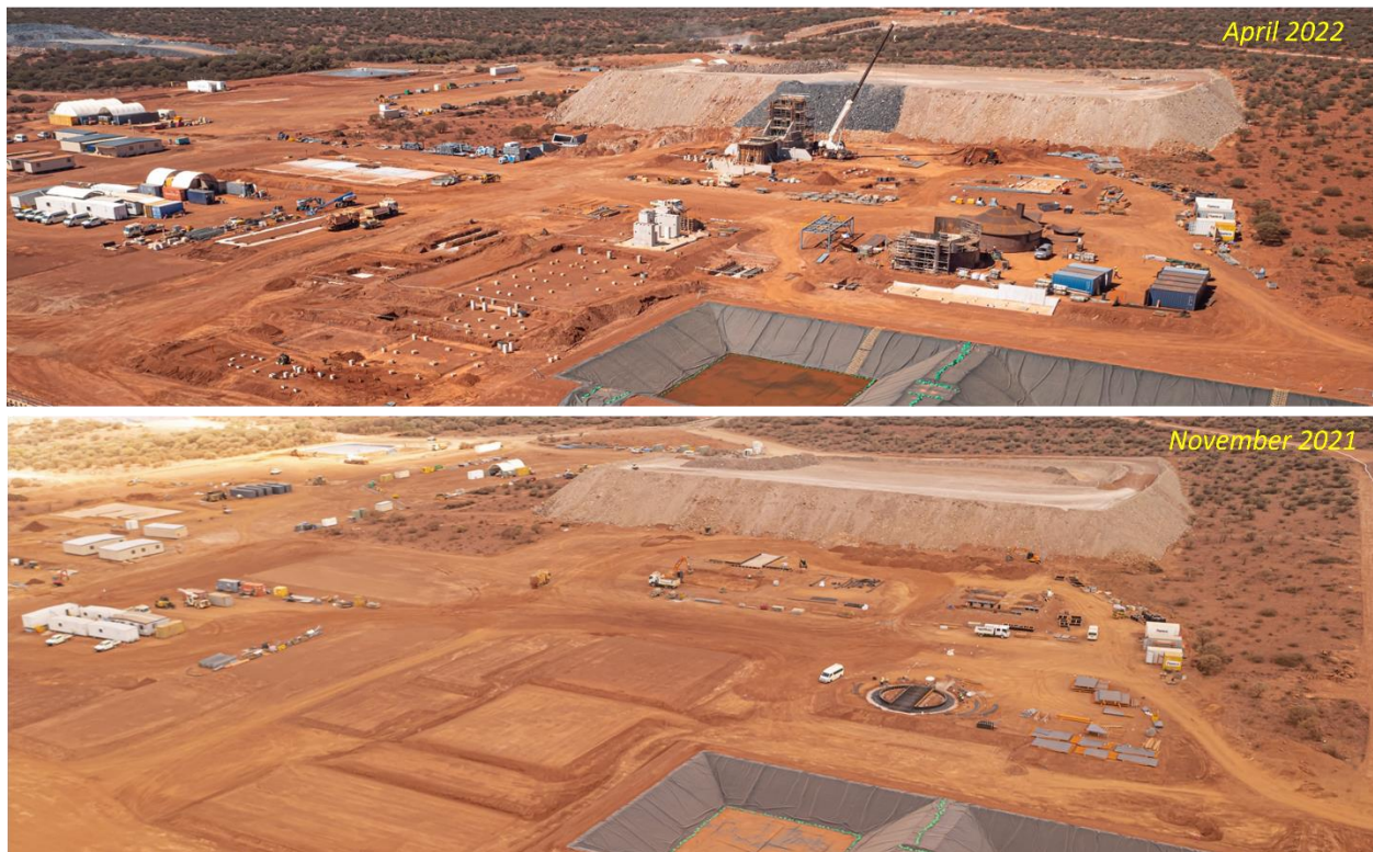
Figure 3. Work progress from November 2021 through to April 2022 at the main Abra plant and infrastructure area looking South.
