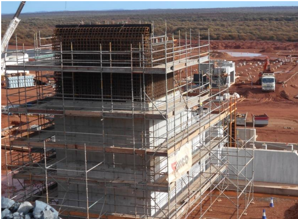
Figure 5. Crusher with formwork and rebar in place prior to third concrete lift (now complete).
