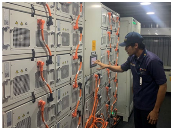
450kWp solar system fully commissioned
