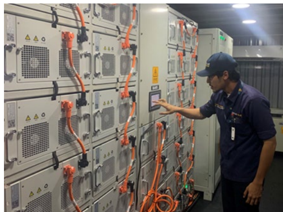
450kWp solar system fully commissioned
