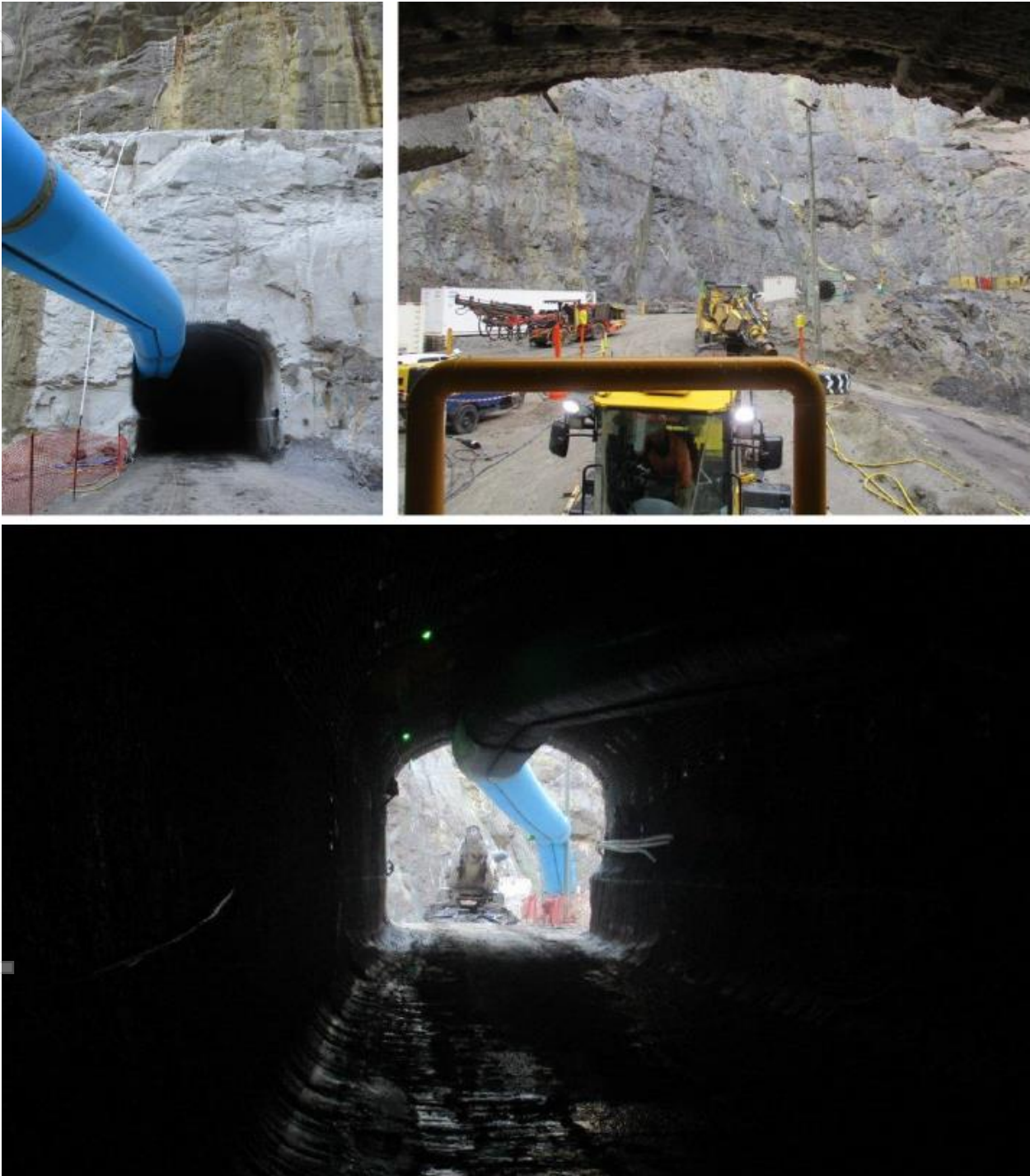
Figure 2 Portal complete (LHS) and view looking out from inside the portal (RHS) and view from within the decline (lower image)
