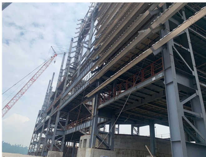
Base of ONI Electric Furnace
