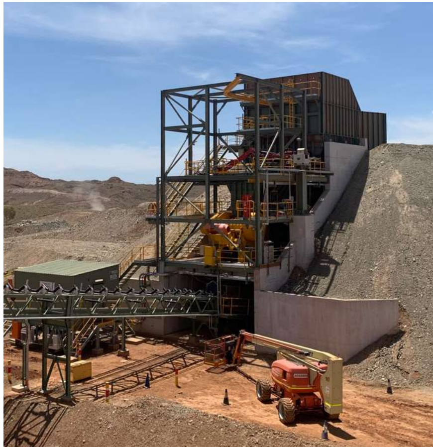
Figure 4: ROM Bin and Crusher
