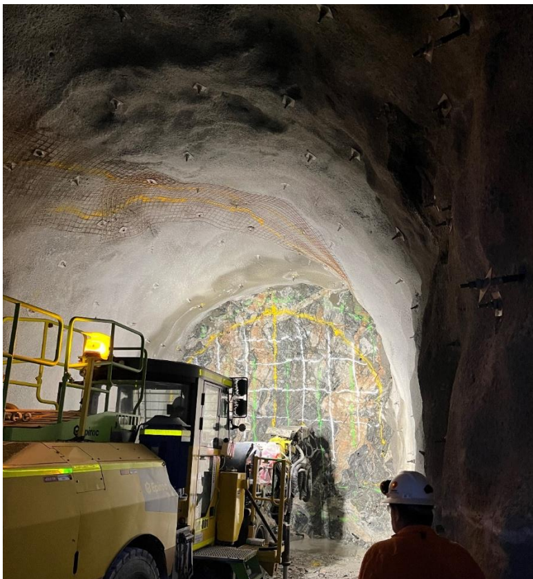
Figure 2: Drilling the face of the MAT in preparation for the next blast
