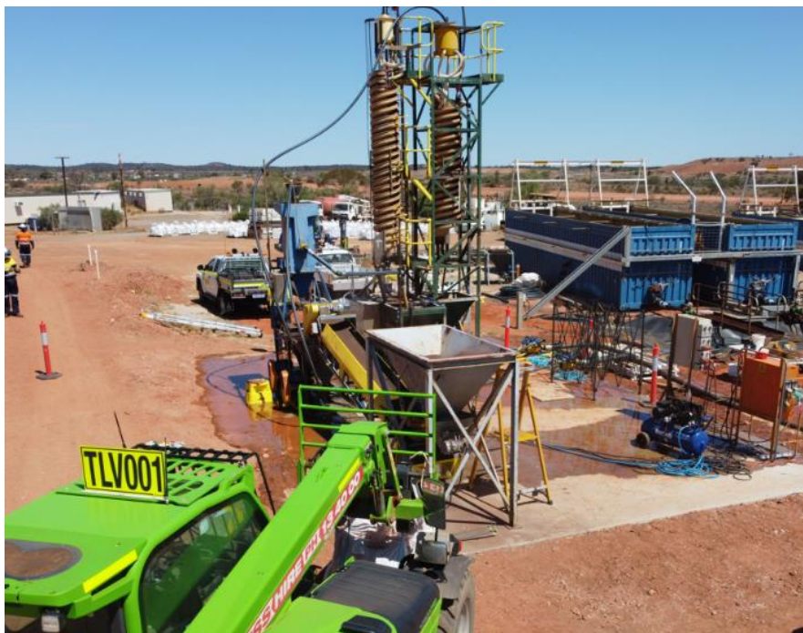
Figure 15– Overview of the Beneficiation Plant
