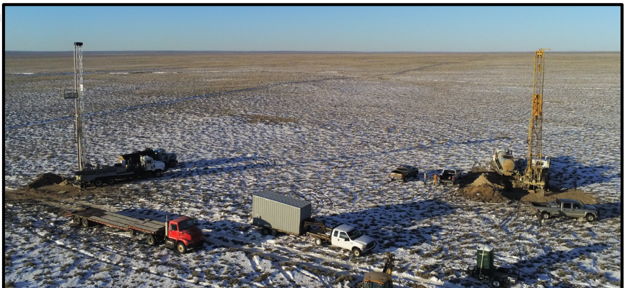
Figure 1. Mud Rotary Drill Rigs Operating at the Thor ISR Uranium Project, GDB, Wyoming USA.
