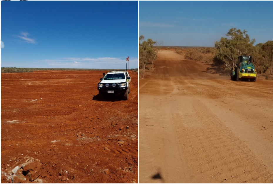
Figure 1 – (Left side) clearing completed for permanent village camp and (Right side) clearing and grubbing of main access road.
