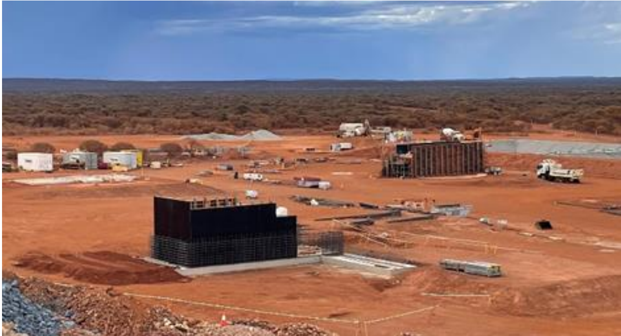
Figure 1 shows some of the Abra processing plant construction activities in January 2022. Concrete foundations being placed in the primary crusher area in the foreground and the fine ore bin (FOB) in the background.
