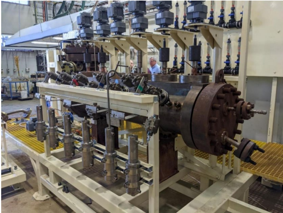
Figure 8. Autoclave for Pilot Plant Phase 1
