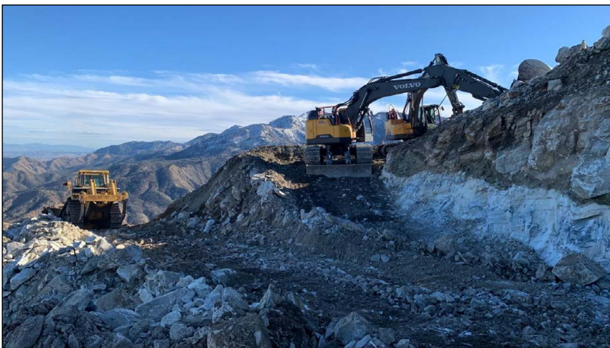
Figure 11 – Earthworks for two additional pads to improve access to southern Talon drill targets.
