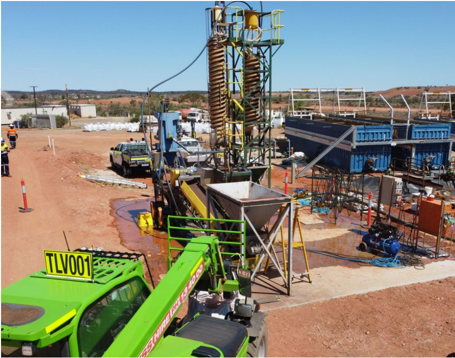
Figure 3 – Overview of the Beneficiation Plant.
