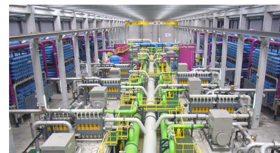
Desalination Plant in Asia
