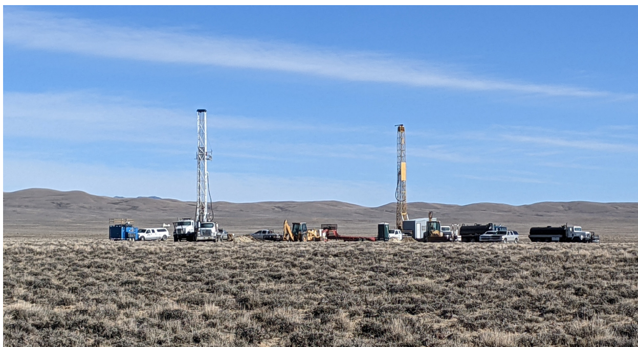
Figure 2. Mud Rotary Drill Rigs (x2), Ancillary Equipment and Support Vehicles at the Thor Project.
