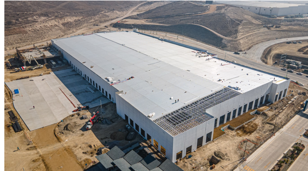
Mexico 3 – Construction progressing well on the third manufacturing facility in Tijuana, Mexico.
