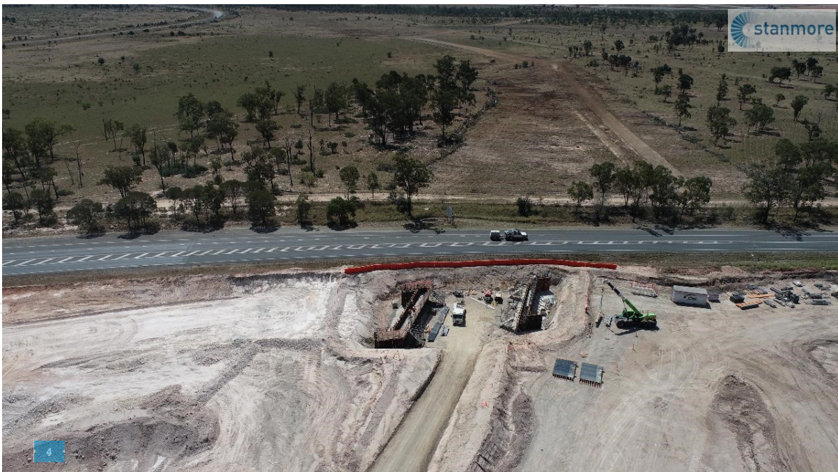
Figure 2: Construction of the concrete underpass bridge next to the Peak Downs Highway
