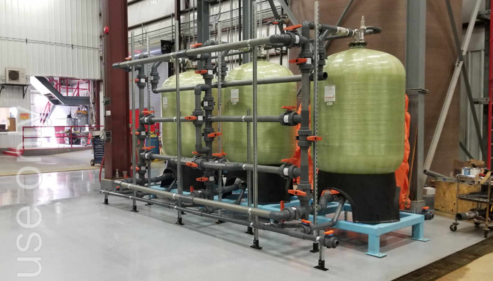
Figure 6: Constructed Ion Exchange Test Columns for MU1A Field Demonstration
