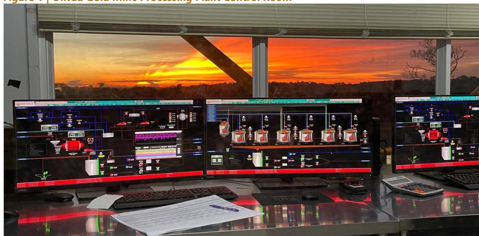
Figure 1 | Okvau Gold Mine Processing Plant Control Room
