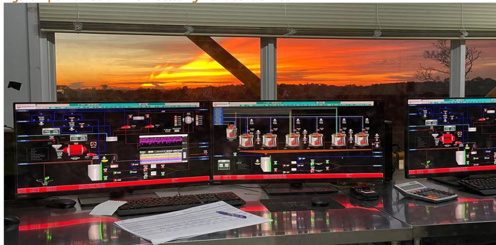
Figure 1 | Okvau Gold Mine Processing Plant Control Room
