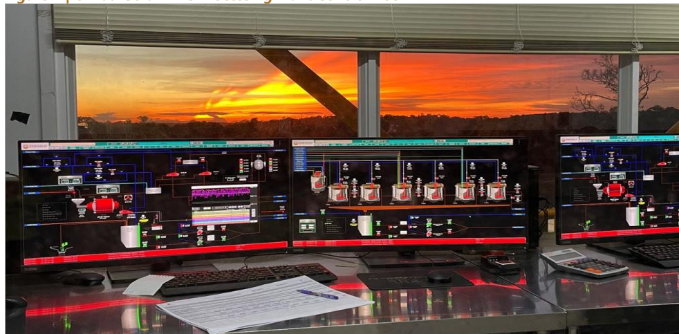
Figure 1 | Okvau Gold Mine Processing Plant Control Room
