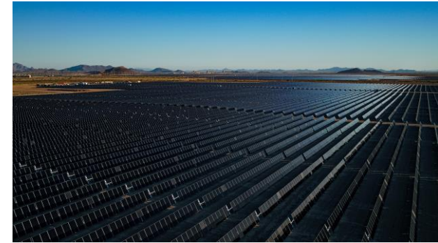
Sun Streams Solar Project, Arizona
